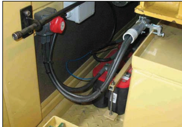
Figure 3-9: Battery package with isolation switch
